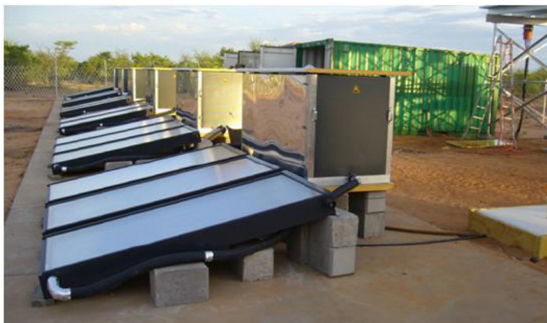
Fig. (13). MSD-desalination systems in Namibia.
